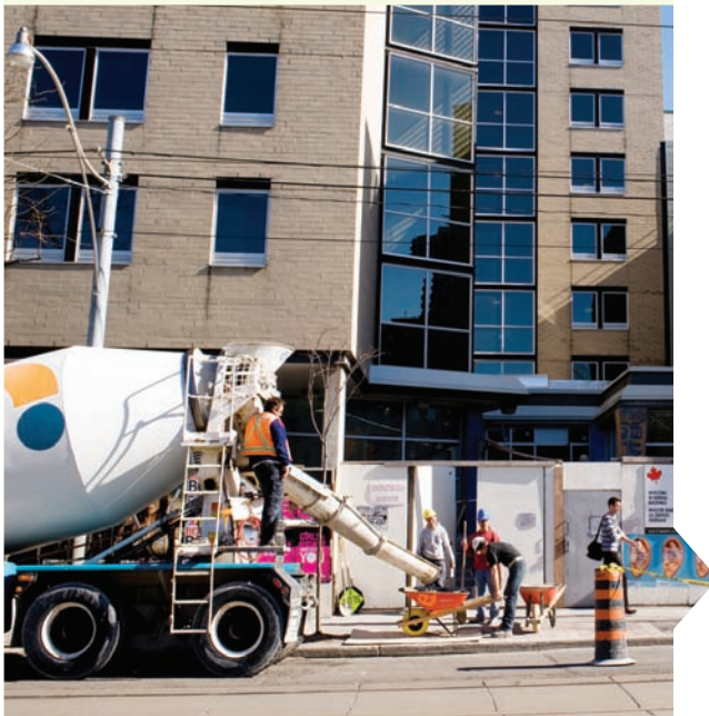
Throughout 2010 and winter 2011, the Queen and Jarvis housing and social service site was under construction. The building is now fully redesigned and rebuilt.
